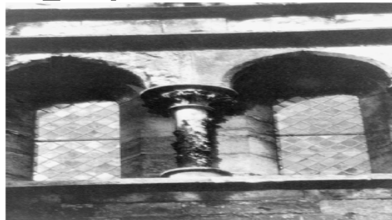
Fig. (6.2). Black crust developed on a column of limestone, Lincoln cathedral, Lincoln, England.
