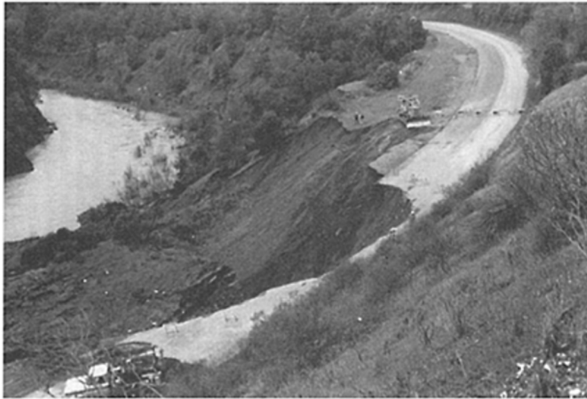
Fig.(5.2). Slope failure at Sonoma County, California.
